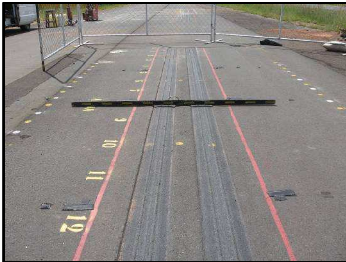
Figure 7. HVS test section showing some rutting (plastic deformation) in the HMA overlay after recent channelised testing with 11R22.5 dual tyres at a road surface temperature of 60 °C.
