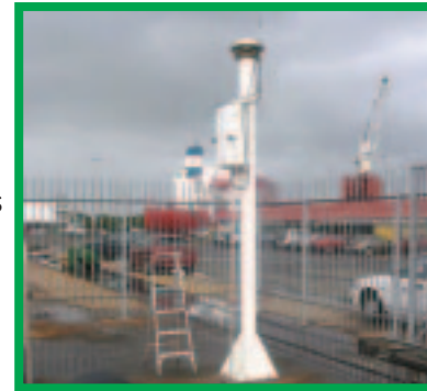
The Richard's Bay GPS antenna on its mast
